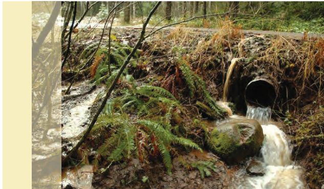
Sediment delivery from culvert near No Whisky Creek
