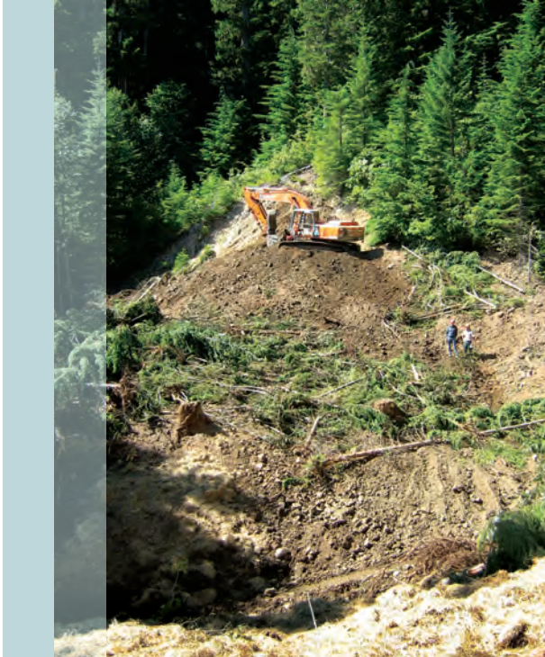
Road decommissioning and stream channel restoration in progress in the Clackamas Ranger District
