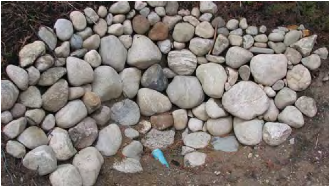
Installation of PVC or steel pipe underneath the tread from drainage basin to sediment trap.
