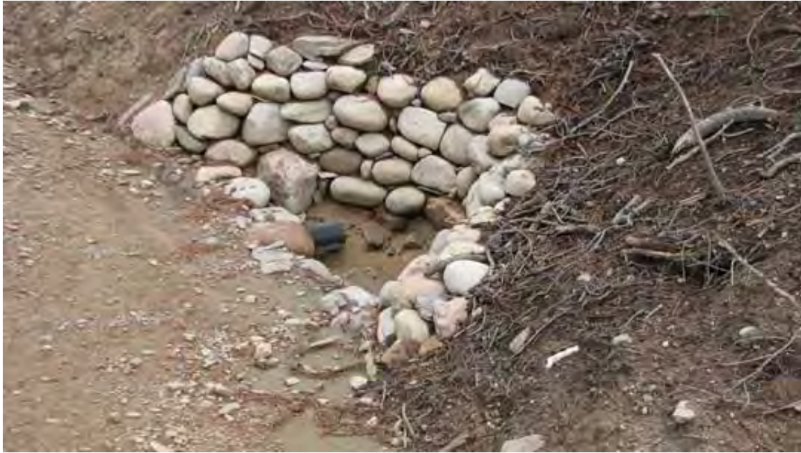
Rock fortify drainage basins and place pipe minimum 3 inches above bottom of drainage basin to allow for silt to drop.
