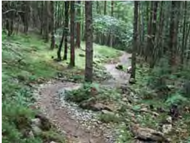
Incorporate grade reversals often throughout trail to improve drainage and guest experience.
