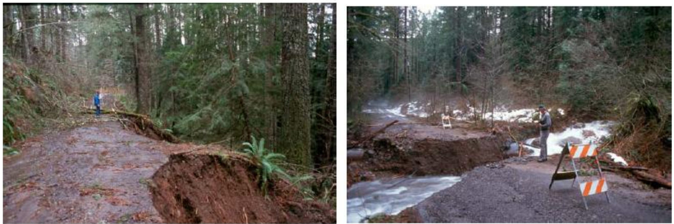
Figure 3.8. Examples of catastrophic fill and culvert failure from the Mt. Hood National Forest Roads Analysis.
