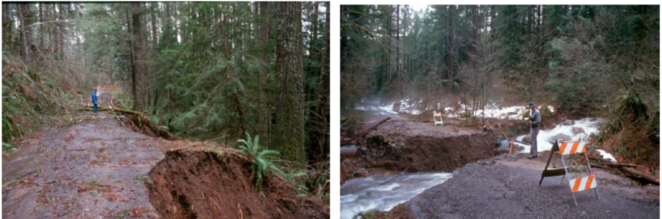
Figure 3.10. Example of catastrophic fill and culvert failure from the Mt. Hood National Forest Roads Analysis
