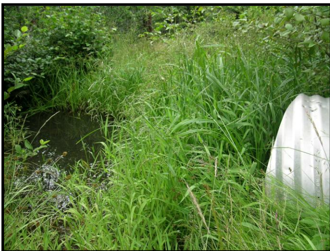
Blocked culvert on Road 17, we documented fish in the pool caused by the culvert, unable to travel further on up the West Fork of Neal Creek
