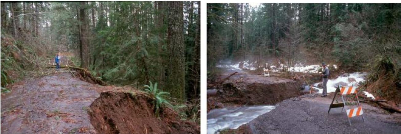
Figure 3.8. Examples of catastrophic fill and culvert failure from the Mt. Hood National Forest Roads Analysis.
